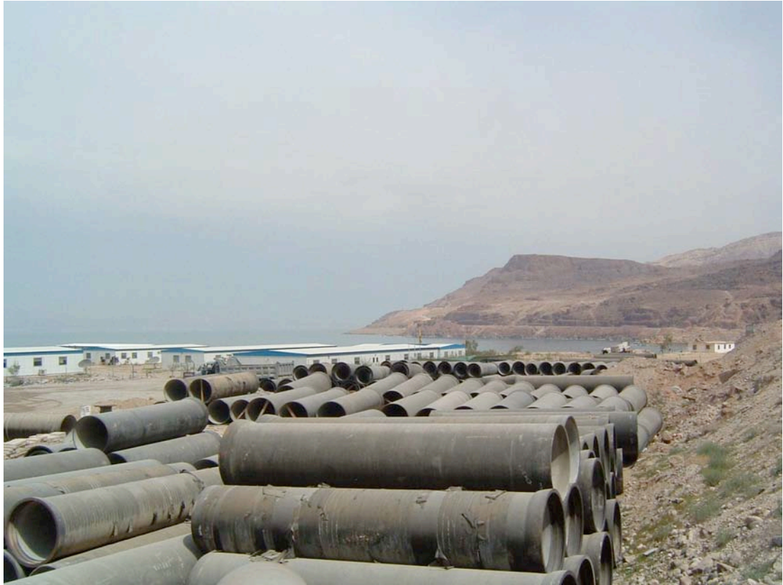
Figure 4: The laying of water pipes in the Jordan Valley close to Wadi Faynan in April 2004, relating to major investment in the management of water for industrial, agricultural and tourism development.
